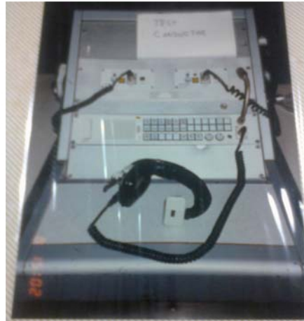
Two Console Mount Stations and an 802 Master Station
