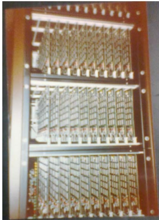
One of the electronics system racks.
